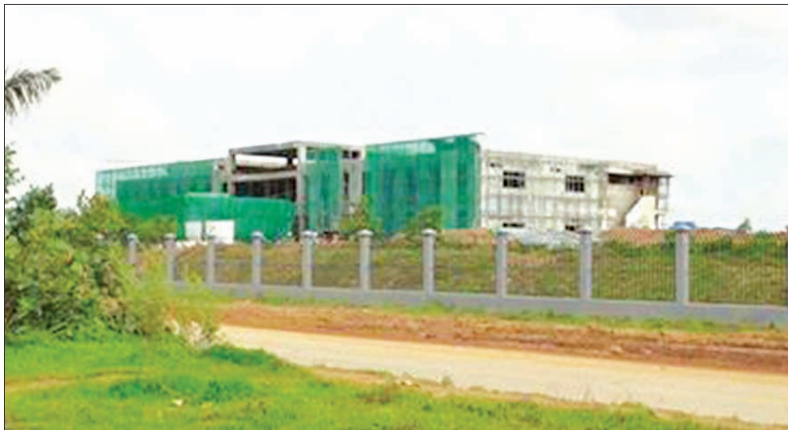
A building is under construction in the Thilawa Special Economic Zone. PHOTO: YE MYINT
