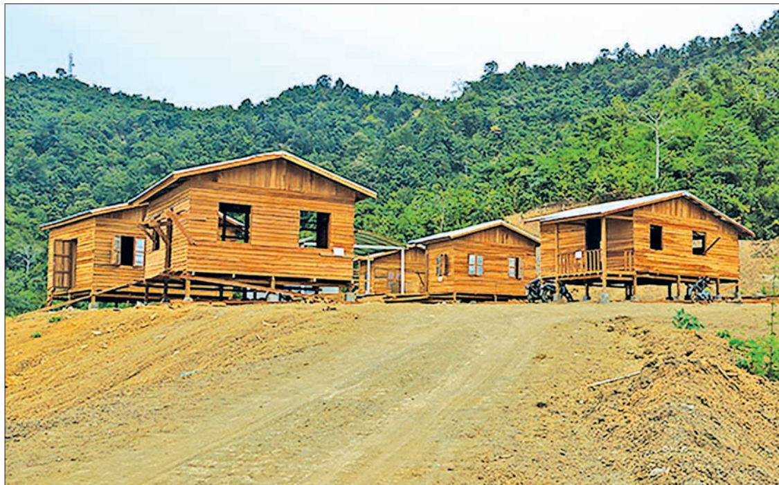
New houses for people in flood-affected areas are under construction in Kalay. PHOTO: JUNINE-KALAY IPRD
