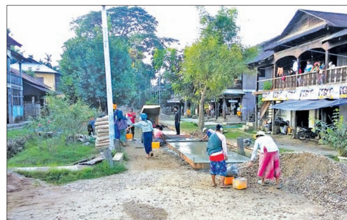
Workers construct a new concrete road to replace an old dirt road in Mawlaik. PHOTO: KYAW PWA
