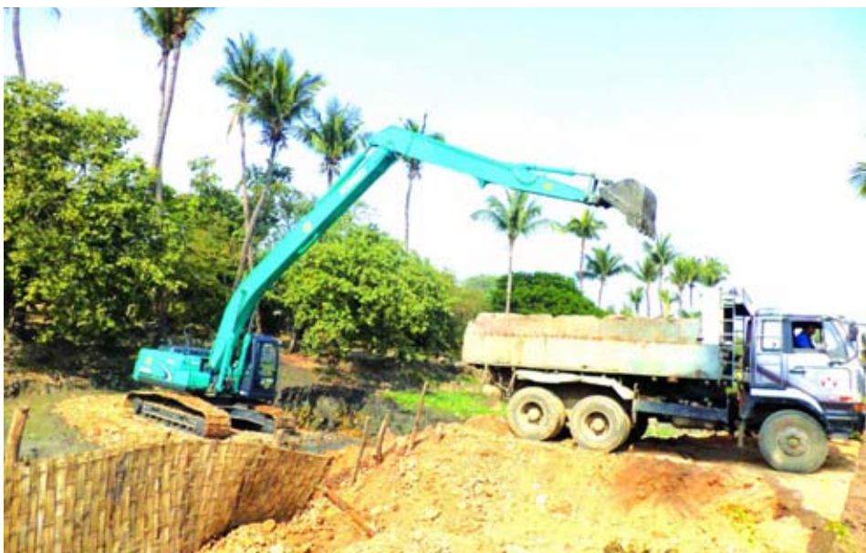
Construction of People's Square in progress in Mahaangmye Township of Mandalay Region.
