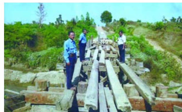
Head of Pyay District Rural Development Department U Min Maung and party inspect reconstruction of Saytaing Bridge between Pauktaw and Agga Villages in Pyay District, Bago Region on 27 December.—KYEMON-HTUT AUNG LWIN
