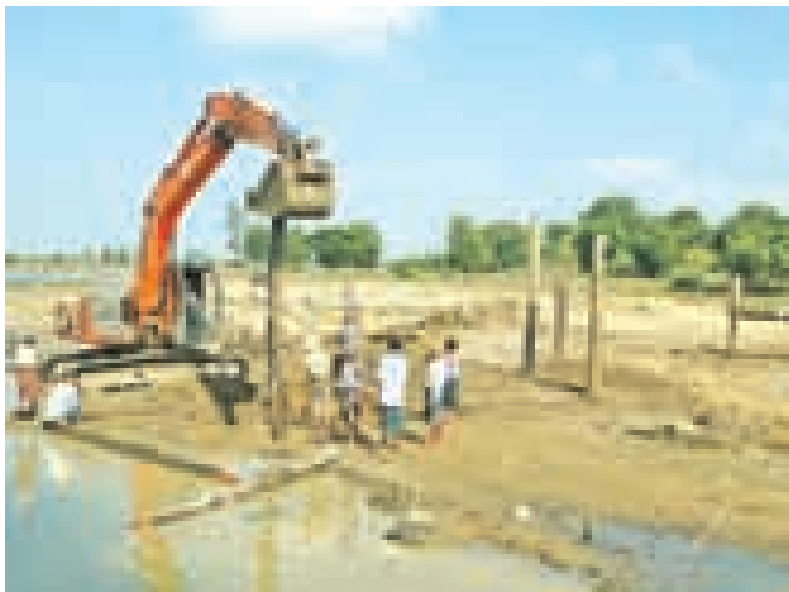
Photo shows construction of a new wooden bridge across Nerinzara River in Kalay.
