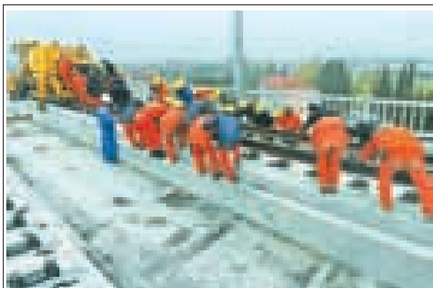
Workers lay tracks at the construction site of Hangzhou-Changsha high-speed railway in Zhuji City, east China's Zhejiang Province, on 10 Nov, 2013. The 920-kilometre high-speed railway linking Hangzhou City and Changsha City, respectively capital of Zhejiang Province and capital of Hunan Province, and designed at a top speed of 350km/h, will reduce the travel time from more than six hours to three hours after it is put into operation in 2014 as expected.—XINHUA
