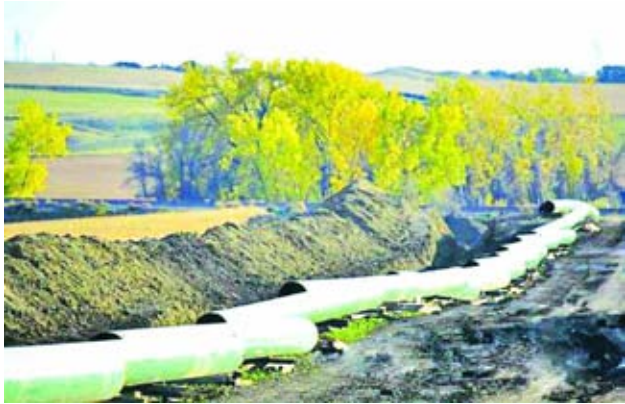
The Keystone Oil Pipeline is pictured under construction in North Dakota in this undated photograph released on 18 Jan, 2012. —REUTERS
