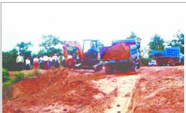
Under the arrangements of Magway Region Government, Region Hluttaw representative U Maung Maung Tin and Township Administrator U Ye Lin Aung together with Township Development Supportive Committee and Township Development Affairs Committee inspect upgrading of the bund of lake in Kyaukpe Village of Minbu Township recently. MMAL-THAN HTAY (IPRD)
