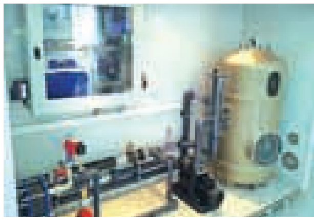
This Prizma pool purification is working in Germany.
