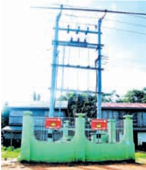
A transformer already installed in Nattalin Township for electrification of local people.
