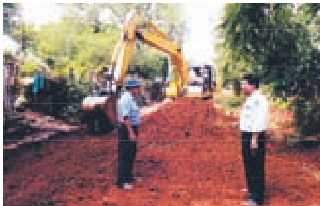
The executive officer and engineer-in-charge of Minhla Township Development Affairs Committee of Magway Region supervise land preparations for construction of 700 feet long and 20 feet wide gravel road for 6 th lane of Ward 6 in Minhla on 18 October.
