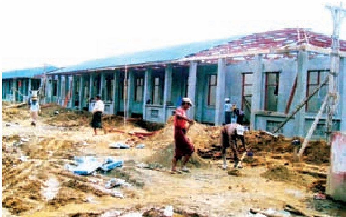
Workers seen at worksite for building new hostels at Sibin guest house in Nay Pyi Taw before XXVII SEA Games.
