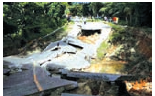
A view of a portion of a damaged highway in Getafe, Bohol a day after an earthquake hit central Philippines October 16, 2013. —Reuters
