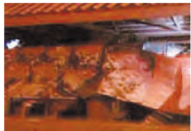
Photo shows damages caused by bomb blast.
