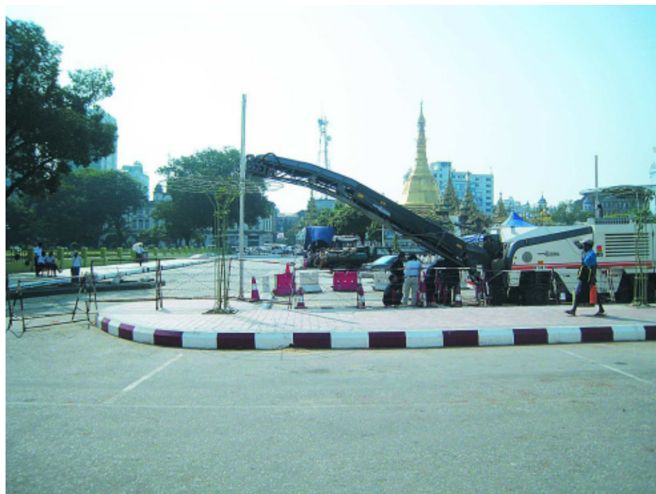
Yangon City Development Committee undertakes development tasks and upgrades the streets around Maha Bandoola Park and places in front of City Hall with the use of heavy machinery for keeping the city neat and tidy to enable the local people and tourists to enjoy pleasant scenes of downtown Yangon.— KYEMON-U SHEIN
