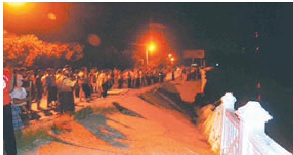
Photo shows collapse of eastern corridor at Meiktila Lake.
