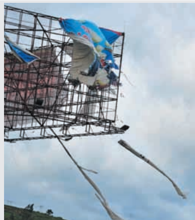
A billboard is damaged by gales in Fuding City, south-east China's Fujian Province, on 6 Oct, 2013. —XINHUA
