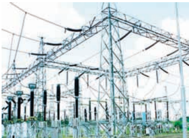
Photo shows a sub-power station.
