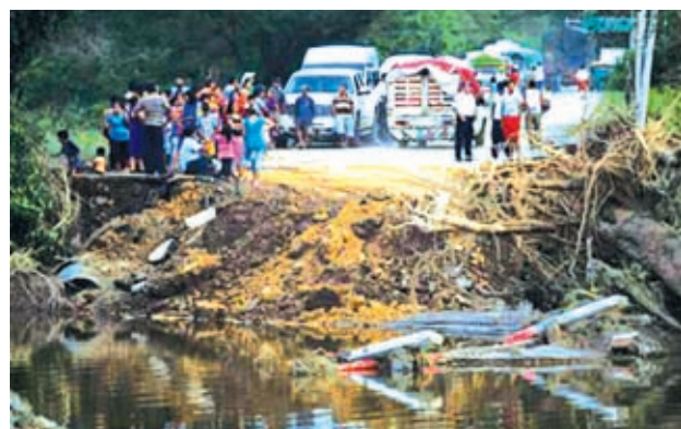
People get out of their cars and gather near a portion of the road collapsed by heavy rains in San Cristobal de Vega in Oaxaca state, on 16 Sept, 2013.
