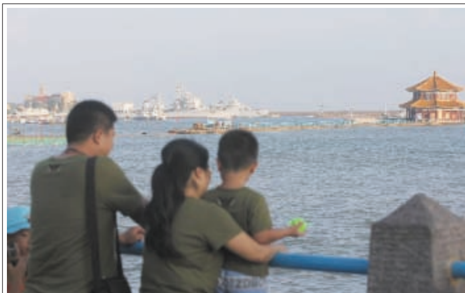
Photo taken on 22 Aug, 2013 shows the Zhanqiao Bridge being under repair in Qingdao City, east China's Shandong Province. A renovation work has been started to repair the Zhanqiao Bridge, a landmark for Qingdao, since part of the bridge was hit and destroyed by thunderstorms and waves on 27 May. The renovation work is expected to be finished by October this year.—XINHUA
