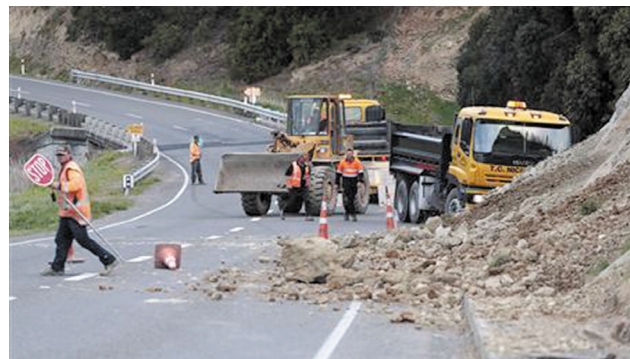
Workmen clear rubble from a road after the side of a hill collapsed after an earthquake on the outskirts of the town of Seddon in the Marlborough region on New Zealand's south island on 16 Aug, 2013.
