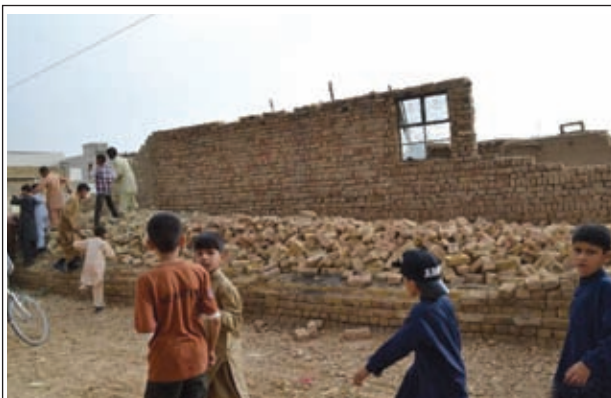
Pakistani children gathered around a fallen house wall in southwest Pakistan's Quetta on 11 Aug, 2013. At least 15 children were injured as the house wall collapsed due to rain in Quetta on Sunday, local media reported.—XINHUA
