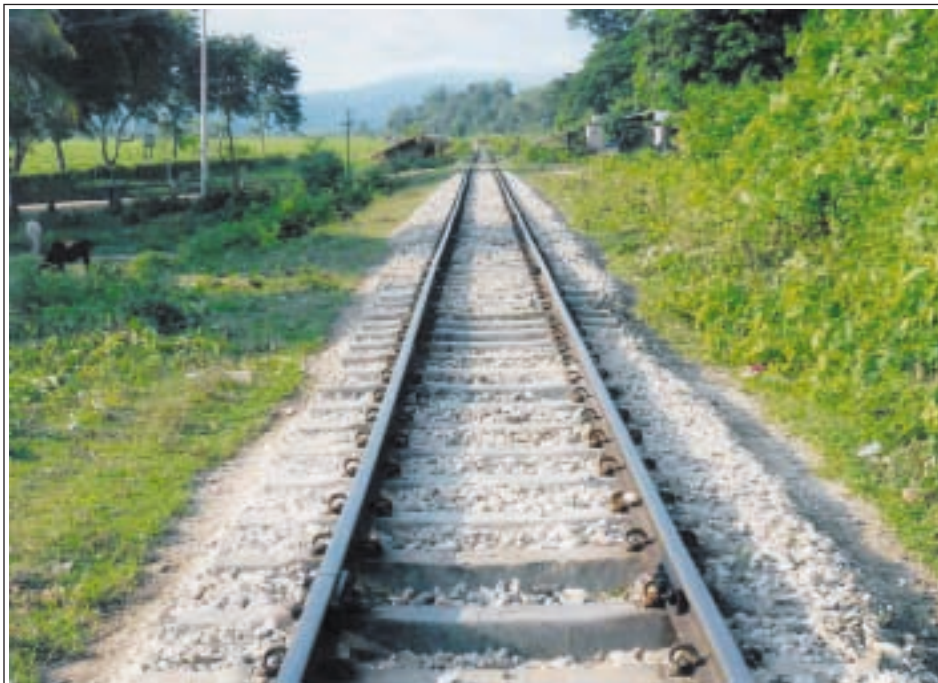
Rail tracks are under maintenance between Mawhan and Kardu railway stations in Mohnyin Township for convenience and safety of trains and passengers.—NLM-001
