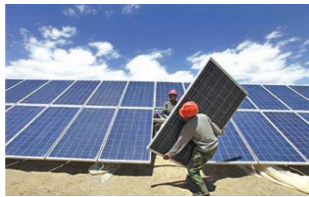
Workers install a solar panel in Jiuquan, Gansu Province, in this on 14 July, 2013 file photo.
