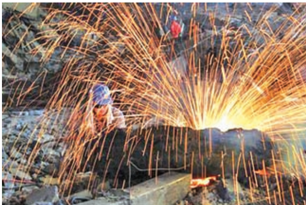
A labourer cuts scrap steel at a factory of Dongbei Special Steel Group Co, Ltd, in Dalian, Liaoning Province on 24 July, 2013.—REUTERS
