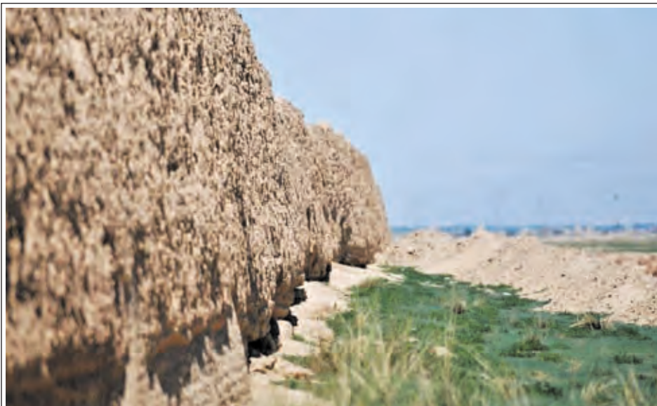
Photo taken on 19 July, 2013 shows the Great Wall in Shandan County, northwest China's Gansu Province. This year, the local authorities has allocated more than 30 million yuan (about 4.89 million US dollars) for the protection of the Great Wall in Shandan County, which was built in the Ming Dynasty (1368-1644) and has a length of 88 kilometres. —XINHUA
