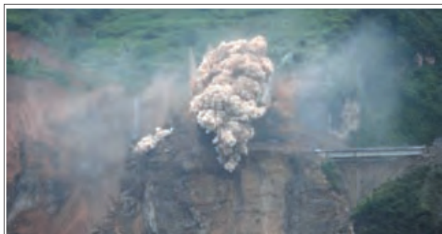
Photo taken on 18 July, 2013 shows the blasting site above a barrier lake in Sanjiao Township of Hanyuan County, southwest China's Sichuan Province. The blasting is conducted to remove dangerous rocks and then dig channels to discharge the floodwater of the barrier lake. The lake was formed after a landslide and continuous rainfall, threatening residents downstream in Sichuan.—XINHUA
