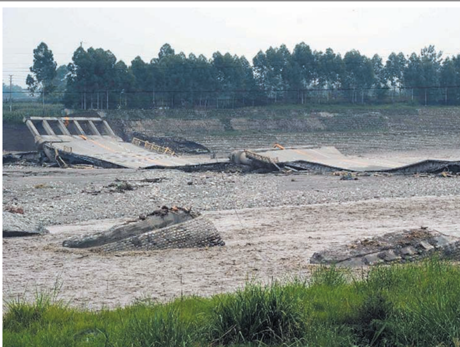
Photo taken on 11 July, 2013 shows the collapsed Chuanxi Bridge in Junyue Town of Pengzhou City, southwest China's Sichuan Province. Rainstorms battered the region these days, and the fast flow of the river water brought damages to the bridge. The damages had been found in time and the traffic had been controlled. No casualties were reported in the accident.
