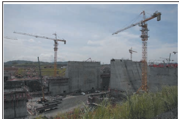
Employees of the expansion project of the Panama Canal work on the new set of locks in the Cocoli sector, in Panama City, capital of Panama, on 10 July, 2013. It's expected that the Atlantic side of the expansion will be finished by December 2014, and the Pacific side mid 2015, according to the local Press. —XINHUA
