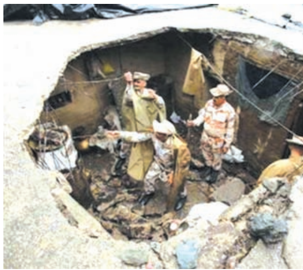
Indo-Tibetan Border Police (ITBP) personnel search for flood victims in a damaged house in Uttarkashi in the Himalayan state of Uttarakhand in this handout photo released on 26 June, 2013.—REUTERS
