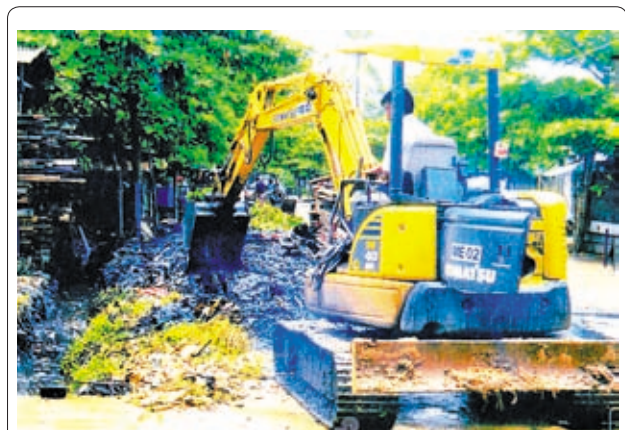
SANITATION CARRIED OUT: Preventive measures against DHF and mosquito are being taken in Myothit C Ward of Insein Township. Max Myanmar Co Ltd dredging drains for proper flow of water while the local people are carrying out sanitation along Midon, Ngasein and Padauk streets on 14 and 15 June.
