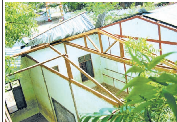
School building of Basic Education Primary School damaged by strong winds.
