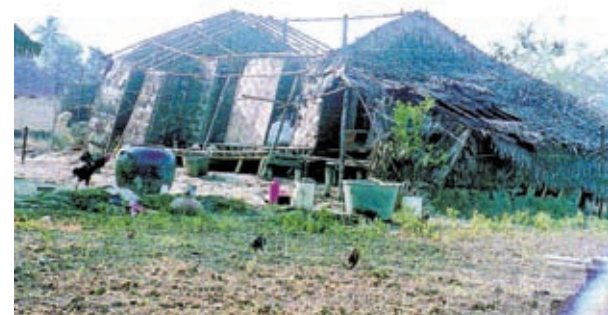
A house flattened by strong winds in Kanpyaung village-tract in Kyauktan Township.
