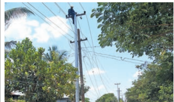
Altogether 12 electricians of Shwepyitha Township Electricity Supply Board install 1400 feet long 6600 volt power line linking 315 KVA transformer at the corner of Pyidawtha and Pathein Road in Ward 10 of Shwepyitha Township on 10 May.
