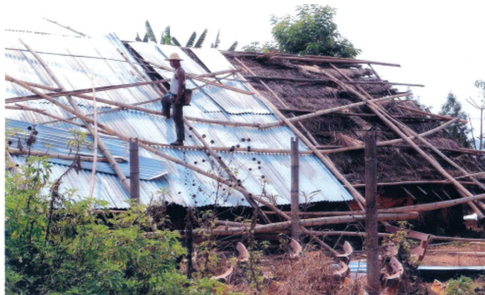
A house collapses in strong winds that hit Humon Village in Ward 12 of Lashio at 6.30 pm on 22 April and at 3.15 pm on 23 April. Due to strong winds, CI sheets of some houses were blown off, trees fell down and power and telephone lines cut out in Lashio.—KYEMON
