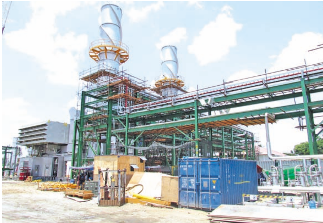
Photo shows 50-MW gas power plant project under construction in the compound of Hlawga gas power plant.
