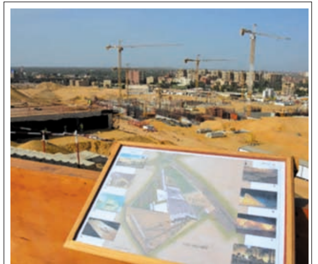
Photo shows the construction site of the Grand Egyptian Museum near the Great Pyramid of Giza on 3 April, 2013. A plan of the museum is seen in the foreground. The Egyptian government said the same day it will solicit a $1 per night donation from foreign tourists at hotels in a campaign to gather money for underfunded construction of the new museum.
