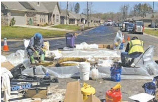
Workers scrub crude oil from their boots in the Northwoods subdivision where an ExxonMobil pipeline ruptured in Mayflower, Arkansas, on 1 April, 2013.
