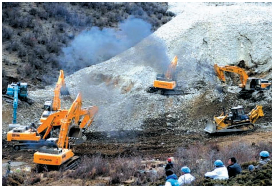
Photo taken on March 29, 2012 shows the scene where a large-scale landslide hit a mining area in Maizhokunggar County of Lhasa, southwest China's Tibet Autonomous Region. Dozens of workers from a subsidiary of China National Gold Group Corporation were trapped. The exact number of trapped workers were not immediately known. —XINHUA
