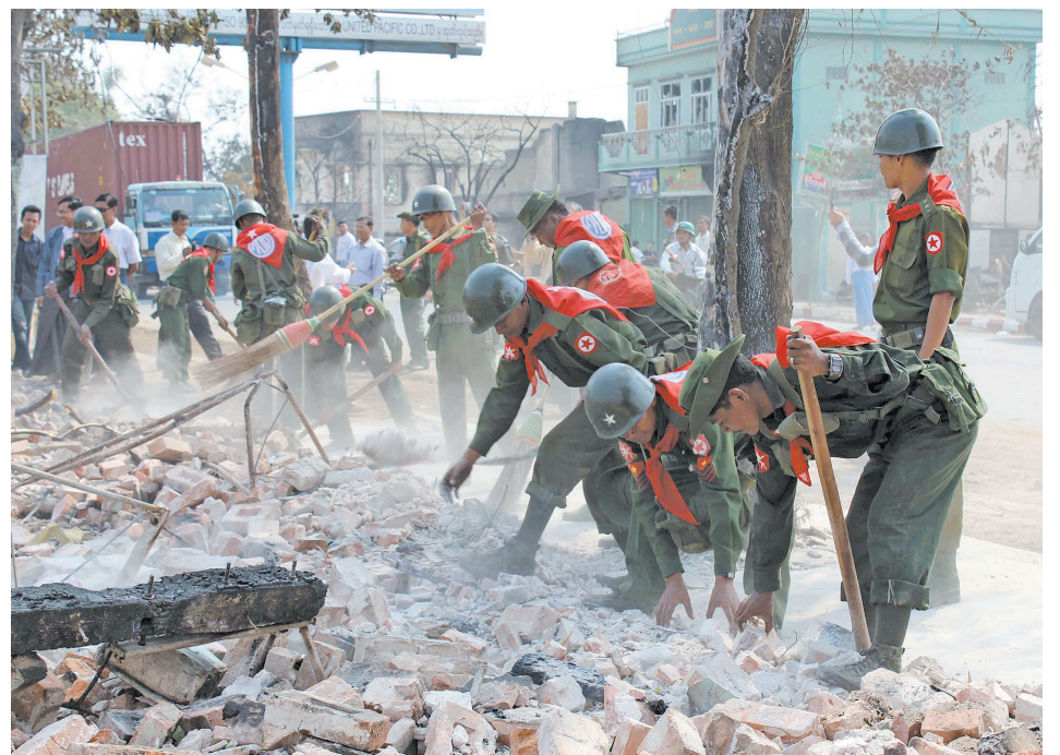
Photo shows Tatmadawmen making rehabilitation works in Meiktila Township. (News on page 8)—MNA
