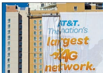
Workers put up a banner advertisement for AT&T on the side of a hotel as they prepare for International CES show in Las Vegas, Nevada on 4 Jan 2013.—REUTERS
