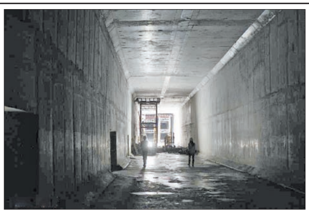
Employees work at the construction site of a new lock for the Panama Canal's widening project in Colon on 19 March, 2013. The new lock is expected to be completed and operated in April 2015, the project's Director General Bernardo Gonzalez said.—XINHUA
