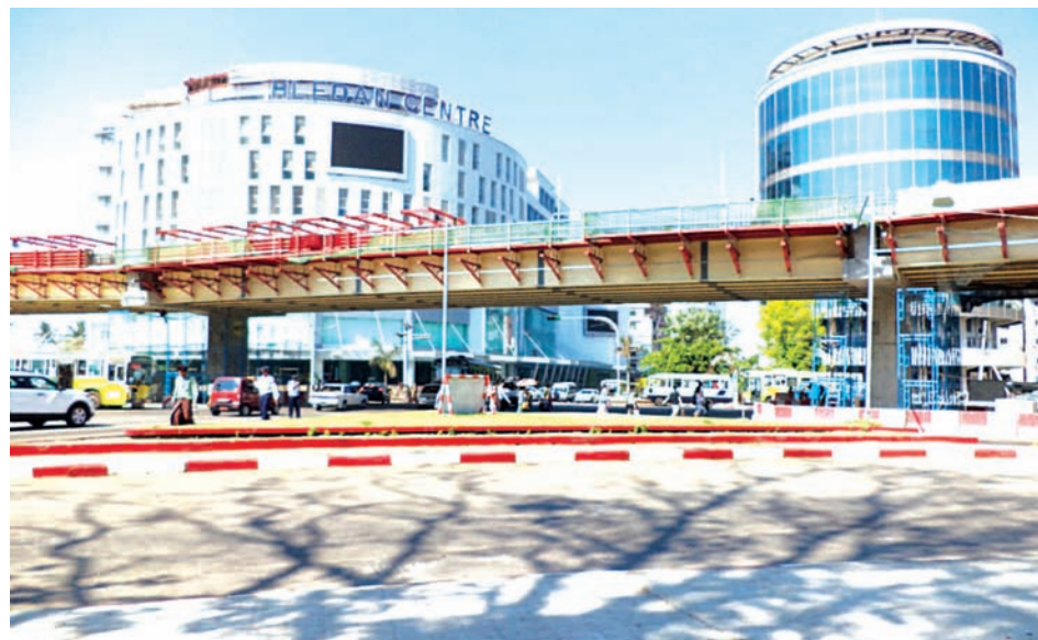
Photo shows Hledan flyover and Hledan Centre which are nearing completion at Hledan junction where a large volume of traffic creates gridlock frequently in Kamayut Township on 18 March.— KYEMON
