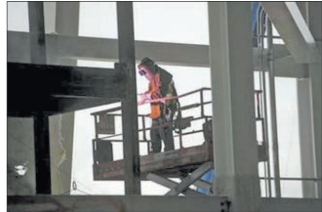
A worker welds a support at Santa Clara Stadium, the future home of the NFL's San Francisco 49'ers, in Santa Clara, California on 6 March, 2013. The stadium is scheduled to open in time for the 2014 NFL season.
