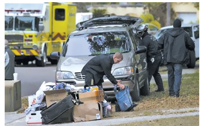
An unidentified man helps to move some of the items salvaged from the house, where Jeffrey Bush was swallowed by a sinkhole, during its demolition in Seffner, Florida on 3 March, 2013.—REUTERS
