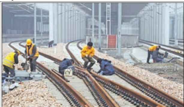
Construction workers and engineers examine rail tracks in the Huzhou Railway Station in Huzhou, east China's Zhejiang Province, on 26 Feb, 2013. The 150-kilometre Hangzhou-Ningbo high-speed railway linking Hangzhou and Ningbo, two hub cities in Zhejiang, commenced its integration test here on Friday.—XINHUA
