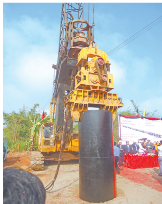
The stake driven ceremony for Myanmar-Laos Mekong River-Crossing Friendship Bridge in progress.—MNA
