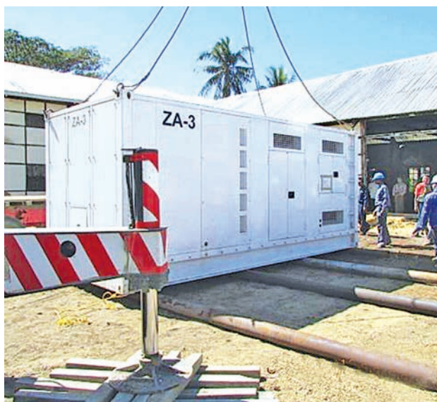
Photo shows a 1000 KVA generator that arrives in Kyaukpyu being moved by crane.
