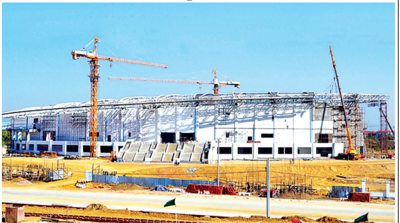
Photo shows progress of Wunna Theikdhi Swimming Pool in Nay Pyi Taw.
