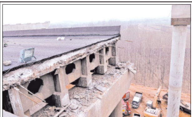
Photo taken on 2 Feb, 2013 shows the bridge collapse accident site in Mianchi County, central China's Henan Province. A part of the expressway viaduct collapsed on Friday morning in an explosion of a truck-load of fireworks. Ten people died and 11 others were injured in the accident. The expressway viaduct, with bidirectional four lanes, opened to traffic in 2001 after three years of construction. —XINHUA
