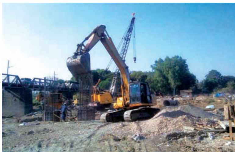
Photo show construction site of Saput creek bridge project in Minbu Township.
