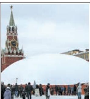
Photo taken on 7 Jan, 2013, shows a temporary dome covering the mausoleum of Soviet state founder Vladimir Lenin in Red Square in Moscow. The dome keeps temperatures inside warmer and allows repair works on the mausoleum to continue even during winter to finish them by the end-of-April deadline. KYODO NEWS
