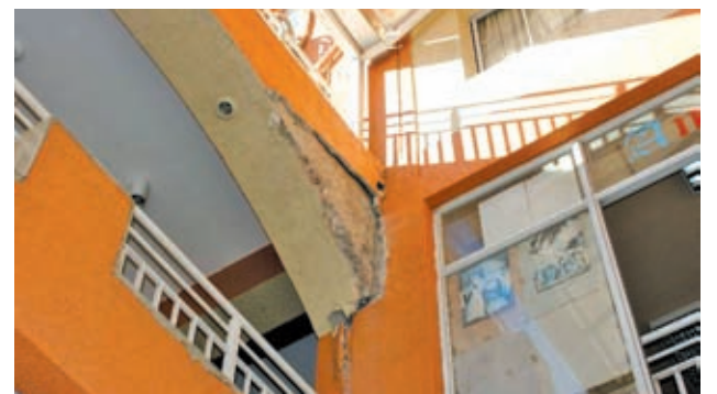
A building suffers structural damage after an earthquake at Copiapo City, Atacama, Chile, on 30 Jan, 2013. A 6.7-magnitude earthquake hit Chile at 4:15 am Thursday (Beijing Time), according to the China Earthquake Networks Centre. The epicenter was monitored at 28.1 degrees south latitude and 70.8 degrees west longitude with a depth of 30 km.—XINHUA
