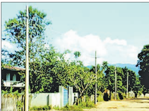
Photo shows progress of substitution of nine-metre long concrete lamp-posts for weather-beaten wooden ones by District/township Electrical Engineer U Nyunt Win and staff with the aim of ensuring safety for dwellers from possible danger of electricity and durability of infrastructure for supply of electricity at Wainwaing village in Monghsat Township of Shan State on 19 January. — KYEMON
