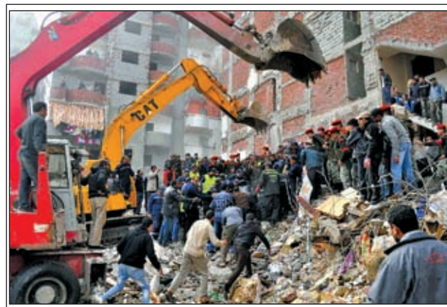
Rescue teams work at a building collapse site in Alexandria, Egypt, on 16 Jan, 2013. The death toll of the building collapse on early Wednesday in Egypt's northern seaside city of Alexandria rose to 16, and 10 injured people have been rescued under the rubble, Health Ministry's spokesman, Ahmed Omar, told Xinhua.
