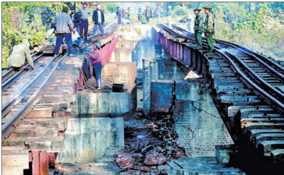
DAMAGED BRIDGE REPAIRED: Two mines went off simultaneously on the bridge No. 436 at Milepost No. 589 between Naba and Indaw Railway Stations on Myitkyina-Man-dalay railroad section and the bridge No. 1 BK on Naba-Katha railroad section on 14-1-2013. The damaged parts were already repaired on 15-1-2013.—MNA
