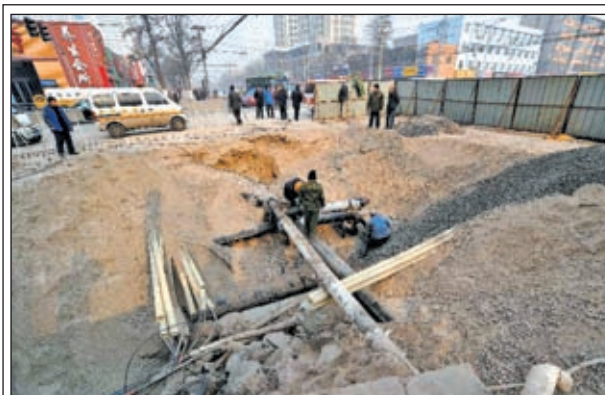
Workers repair the damaged pipelines at the collapsed section of the road intersection of Bingzhou North Road and Bingzhou East Street in Taiyuan, capital of north China's Shanxi Province, on 27 Dec, 2012. The backfilling of the collapsed section has begun, and the damaged pipelines for water and gas supply has been repaired and resumed operation on Thursday, a day after the road cave-in happened. The cave-in left a pit measuring around 3 to 4 meters deep, 15 meters long and 5 meters wide, while damaging pipelines for water, gas and telecommunication.—XINHUA
